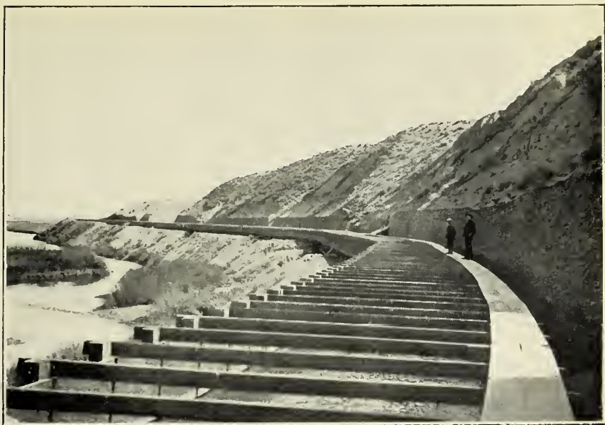
FIG. 1.—FLUME No. 1, KENNEWICK CANAL. SHOWS SIDEHILL CUT THROUGH CEMENT GRAVEL TO FORM BENCH FOR FLUME.
